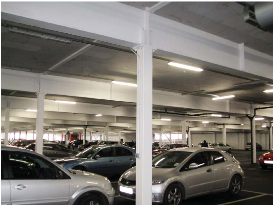
Figure 2: Typical supermarket car park interior steel. Many metres from potential external weathering and in a dry well ventilated environment. Assumes building is water tight.
