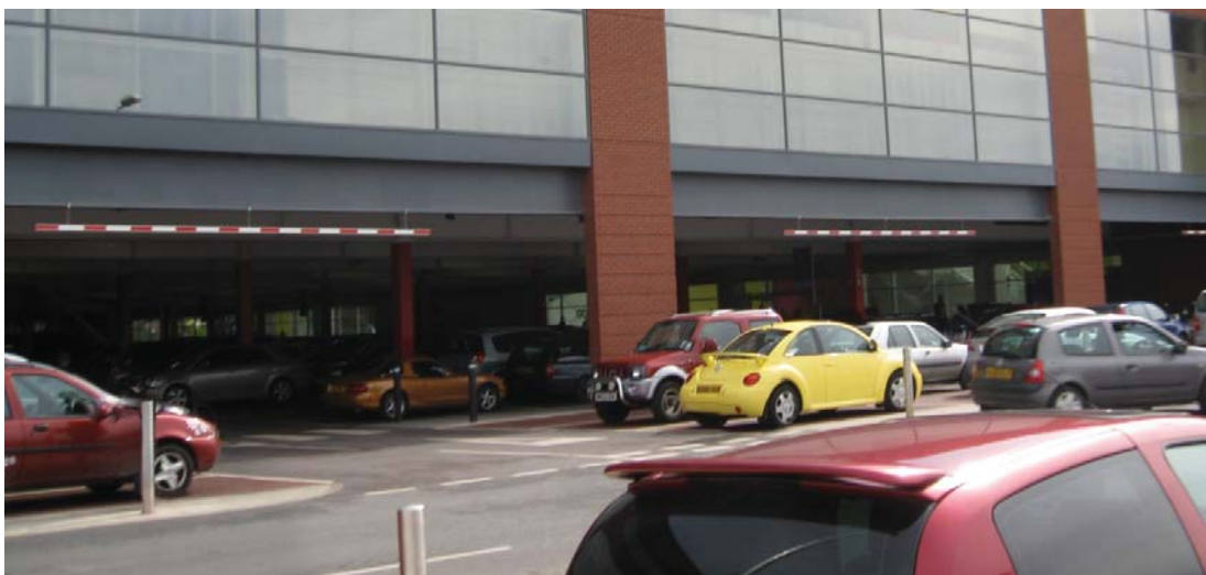
Figure 1: Typical perimeter steel detail that would be subjected to normal weathering conditions.
