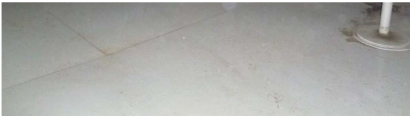
Dura-Plate™ UHS 24-30 mils DFT after nearly 9 years of crude/water immersion
